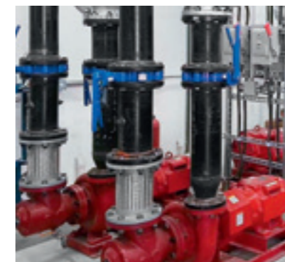
CLOSED-LOOP COOLING WATER, SIKA CORPORATION PLANT LYNDHURST, USA
